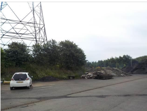
(5) Looking southeast. There are cracks/cuttings in the tarmacadam.
